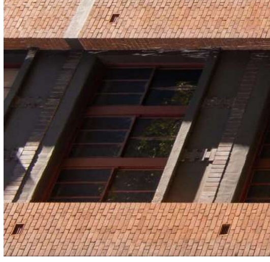
EXISTING FACE BRICK WALL & RECLAIMED TIMBER STRUCTURE REFURBISHED EXISTING NEW HERITAGE PAINT TO RENDER & WINDOW FRAMES
